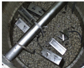
Fig. 5: Corroded SO 2 stripper distributor.
