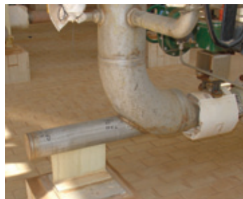
Fig. 1: Dummy pipe support on elbow.
