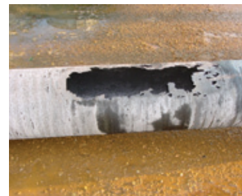
Fig. 7: Pump discharge pipe corrosion.
