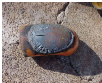
Fig. 2: Slit on elbow. Note the dummy pipe support outline on elbow.
