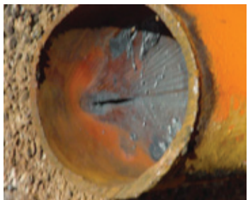
Fig. 3: Erosion-corrosion on elbow.
