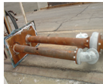
Fig. 6: Hole in pump discharge pipe. Pump shaft column is also corroded.
