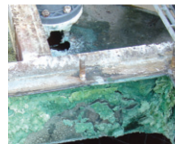
Fig. 8: Stainless steel roof nozzle and pump support beam corrosion.
