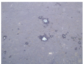
Fig. 4: Sulfate on asphalt roadway coming from the stack.
