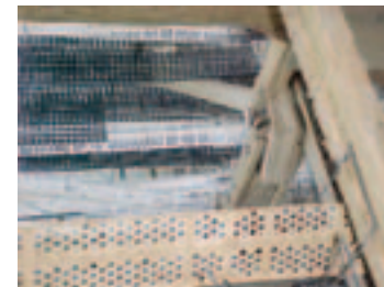
Fig. 5: Broken wooden column inside a cooling tower
