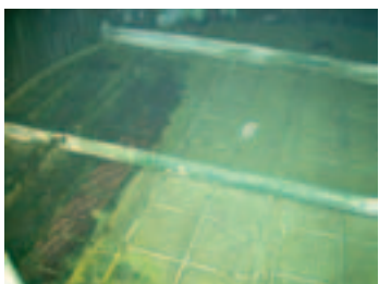
Fig. 2: Drying tower mesh pad corrosion due to loss of absorption efficiency.
