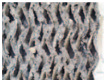
Fig. 3: Clogged bottom section of heat transfer fill.
