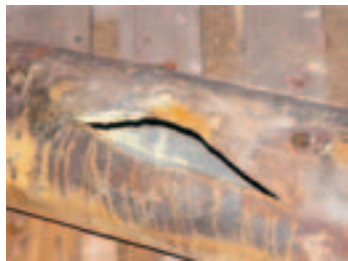
Fig. 1: Thick-lip rupture of 8" sulfur pipe.
