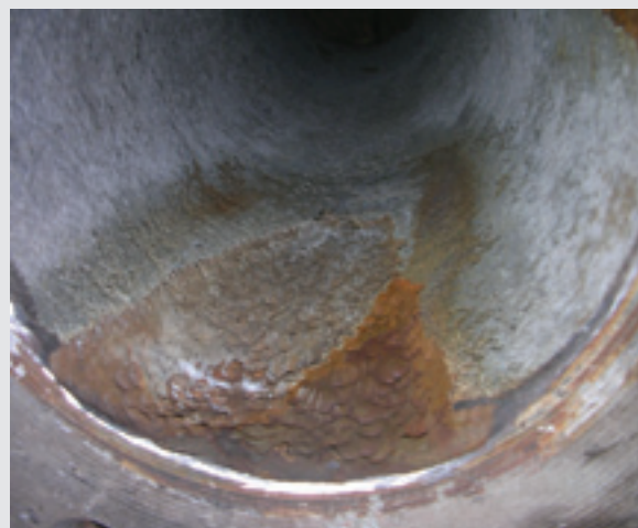
Picture 1: Localized metal loss caused by eddy currents in a ductile iron pipe.
